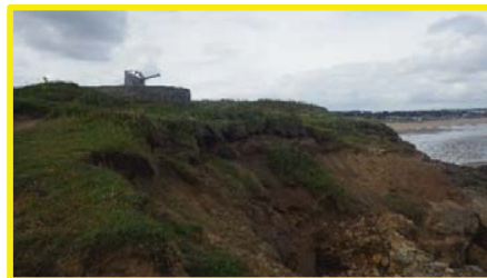
Local slumps in the overlying material at Trow Point.
