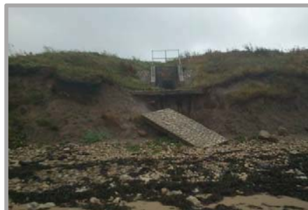
Photo from 2012 report showing failed outfall scour protection south end of frontage.
