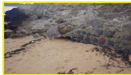
Voids along toe of revetment.
