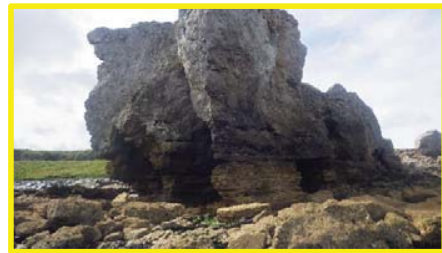
Undercutting of lower levels and caves forming at the base of Target Rock.
