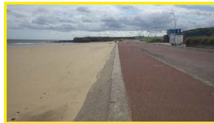
Minor spalling and abrasion to sloping concrete south of lifeguard station.
