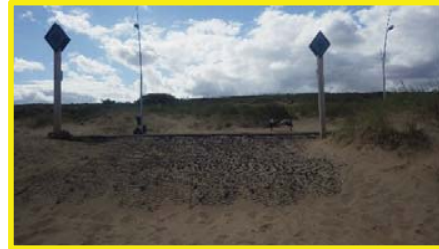
Exposed gabions at access points across dunes.
