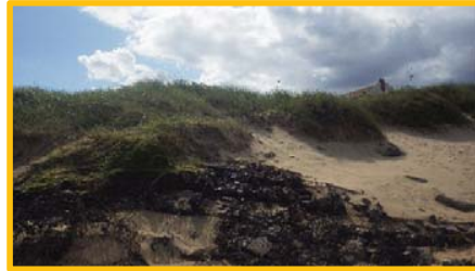
Breaking up of gabions adjacent to ramp at south end of dunes.
