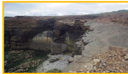
Undermining of concrete defences used to 'plug' caves.
