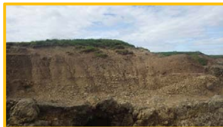
Slippage of soft material.
