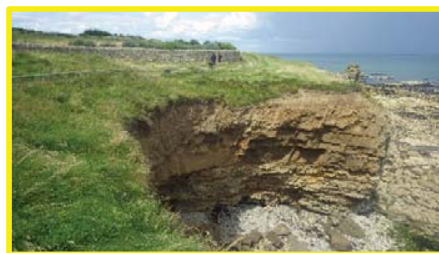
Rock fall bringing cliff face close to coastal path.
