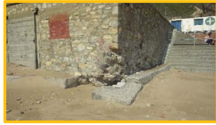
Damage to corner of stone building, vertical cracking.
