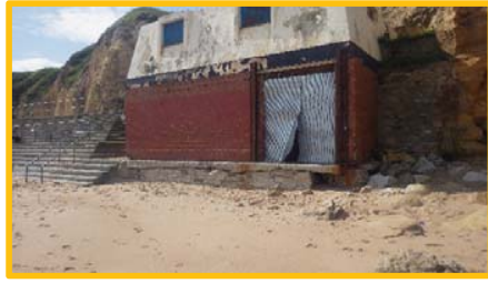
Undermining of structure at disused lifeboat station.
