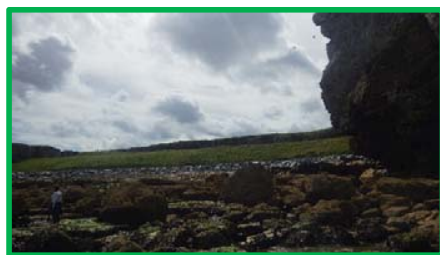
Rock revetment and re-graded slope at Southern Bay in very good condition.
