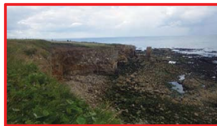
Rock falls and voids at base of cliff south of Lizard Point.
