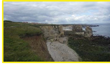
Slippage of soft material and further slumping imminent.
